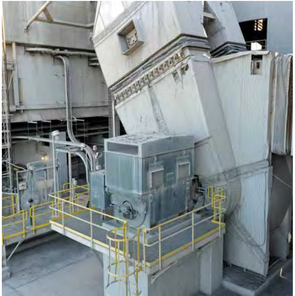
The kiln-induced draft (ID) fan is powered by a 5,000 HP WPII Baldor•Reliance large AC motor. The ID fan is a central element in the clinker production process as raw meal is fed into the kiln and sintered.
